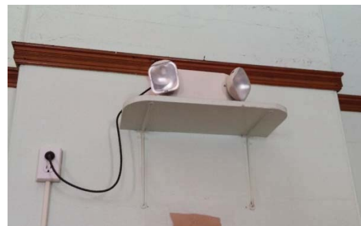
Emergency Egress Lighting
