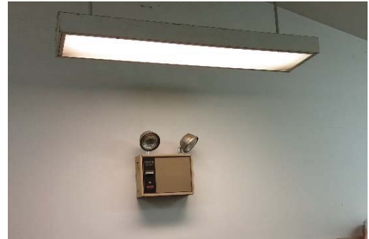
Emergency Egress Lighting
