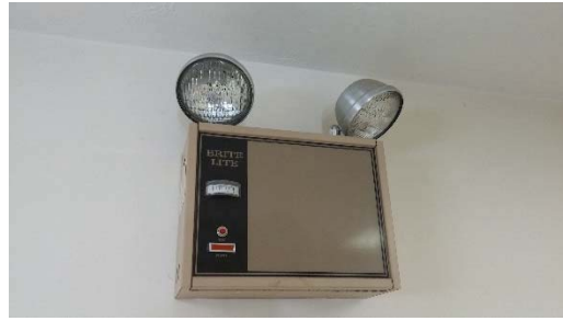
Emergency Egress Lighting
