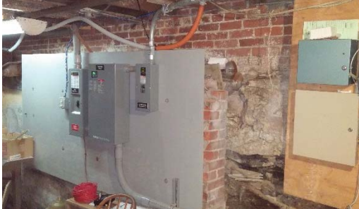
Service Entrance Equipment – 1
