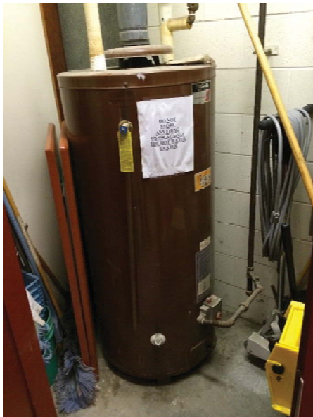
Photo 3: Hot Water Heater
