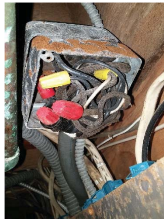
Junction Box / Wiring Sample
