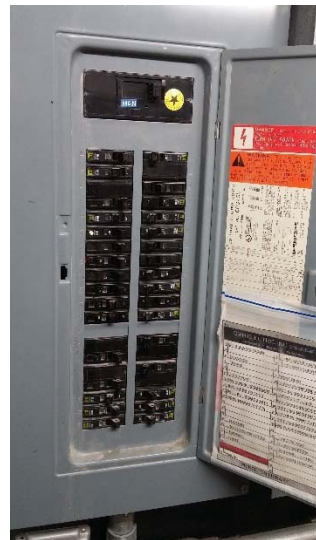
Main Distribution Panel
