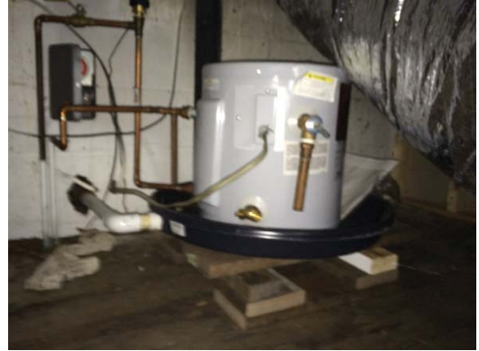
Photo 2: Hot Water Heater
