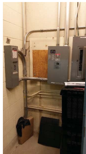
Emergency (Stand-By) Closet
