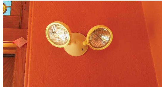
Emergency Egress Lighting
