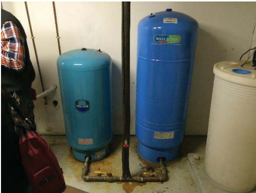
Photo 1: Well Pump Tanks
