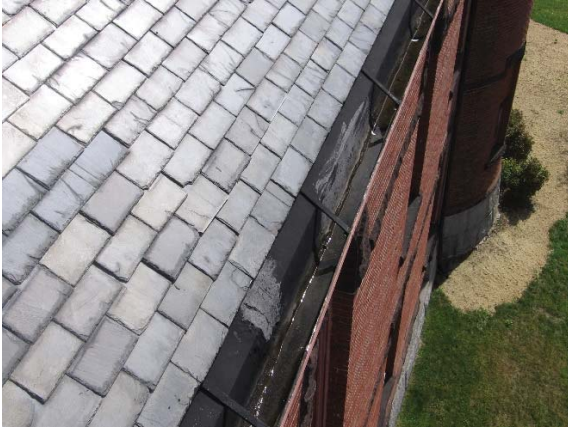
Deteriorated wood gutter lining:
