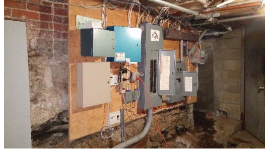
Service Entrance Equipment – 2
