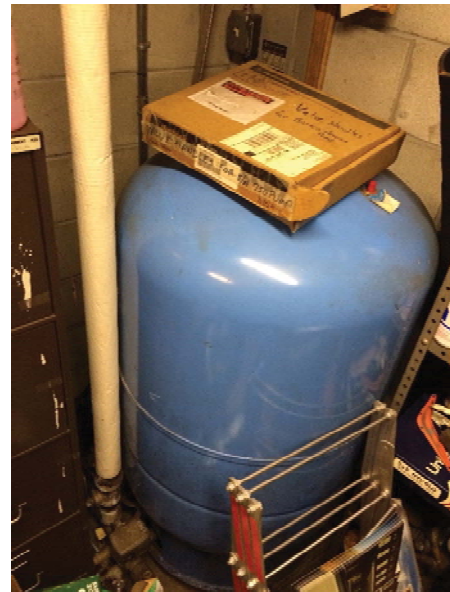
Photo 4: Well Pump Tank
