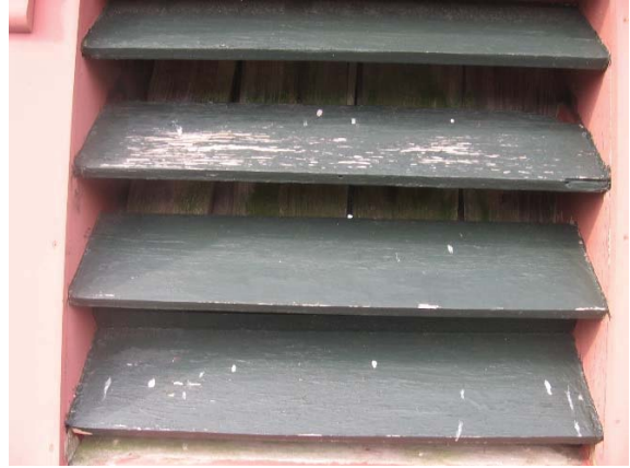
Non-weatherproofed louver at cupola:
