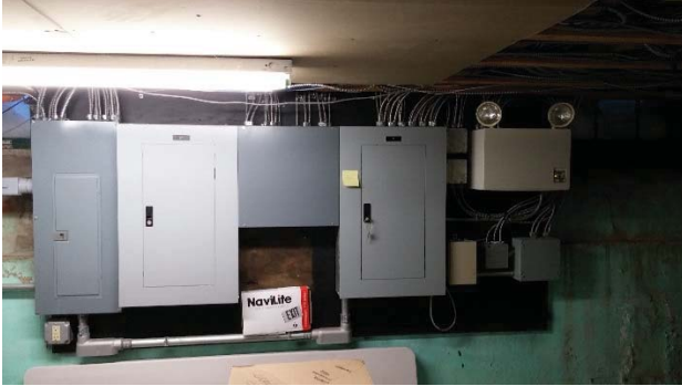
Service Entrance Equipment – Normal
