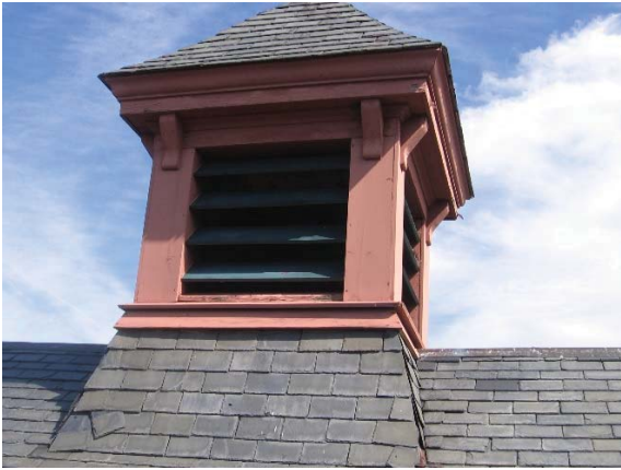
General repairs needed on cupola:
