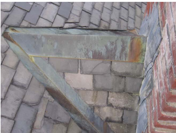
Flashings are in poor condition:
