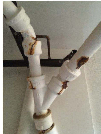
Photo 4: Deteriorating Sanitary Piping
