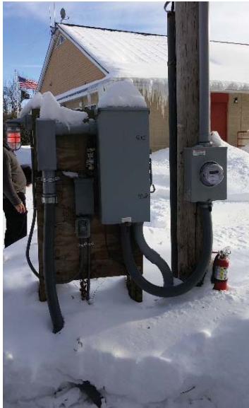
Service Entrance @ Generator
