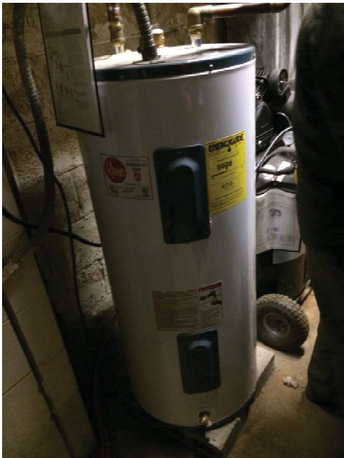
Photo 3: Hot Water Heater
