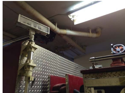
Photo 10: Storm Water Piping
