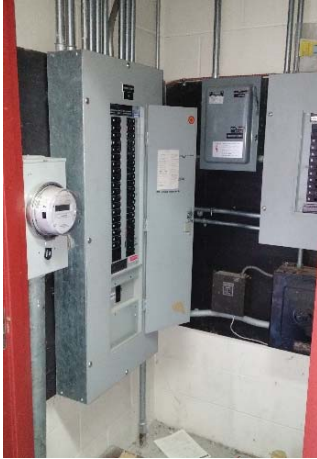
Normal Electrical Room
