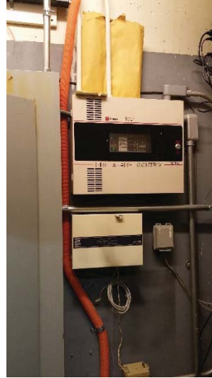
Fire Alarm Control Panel
