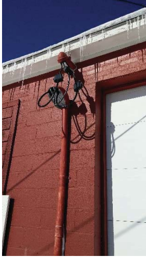
Service Entrance Weather Head
