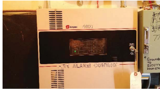
Fire Alarm Control Panel
