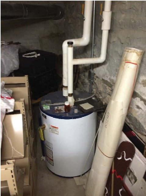
Photo 3: Hot Water Heater
