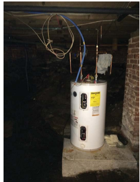
Photo 2 Hot Water Heater
