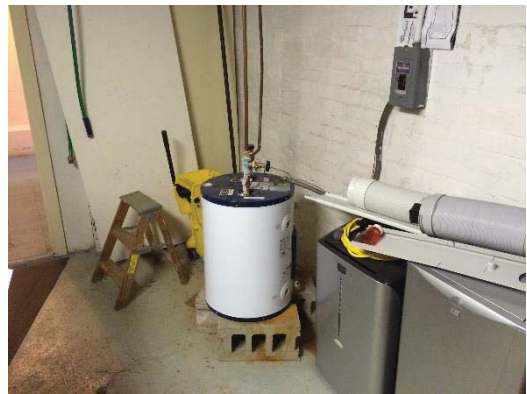
Photo 2: Hot Water Heater
