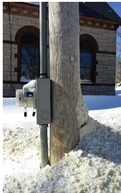
Meter Socket on Utility Pole
