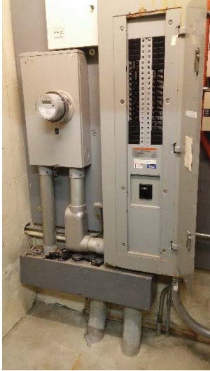
Service Entrance Equipment – Normal
