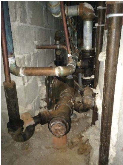
Photo 3: Deteriorating Sanitary Piping
