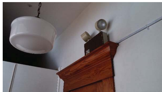
Emergency Egress Lighting
