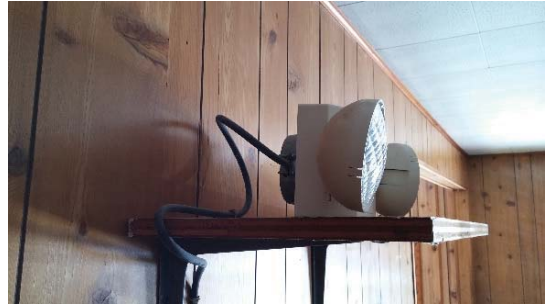
Emergency Egress Lighting
