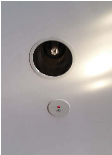
Emergency Egress Lighting
