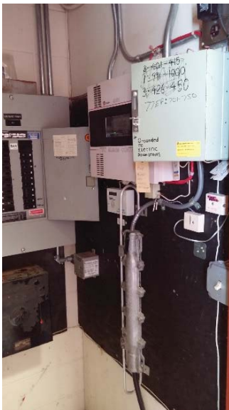
Normal Electrical Room
