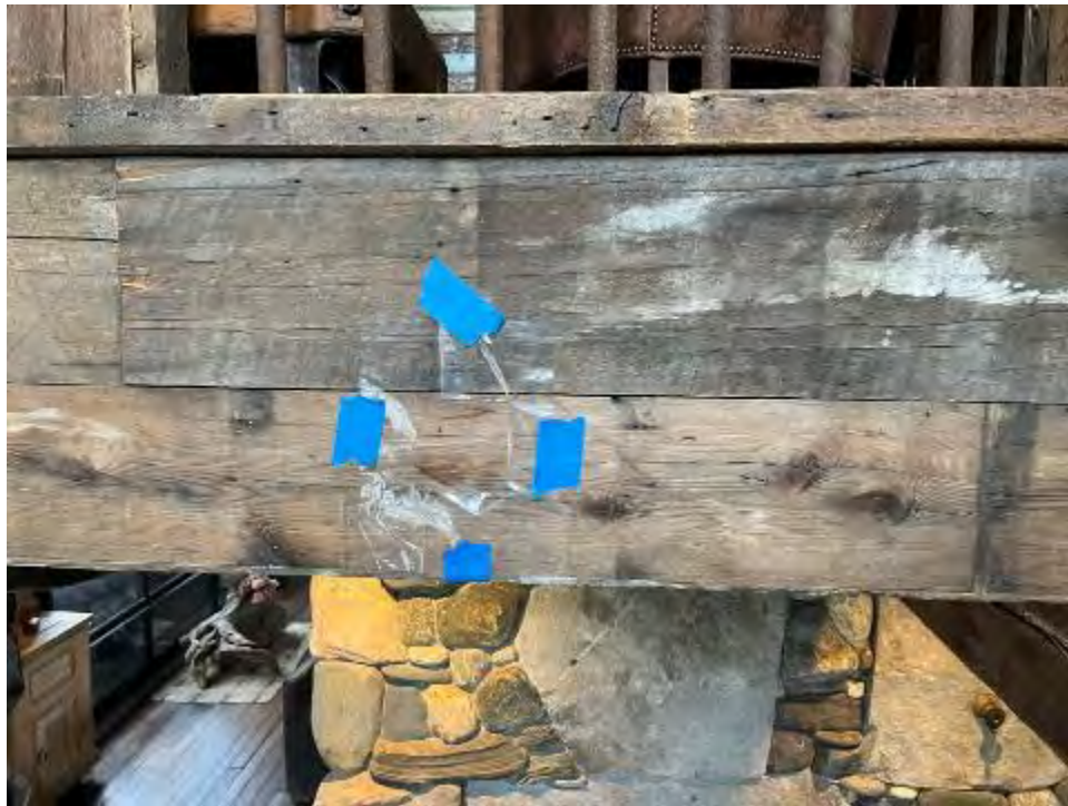
SCENE: View of wipe sample location WP-08 collected from the second floor foyer/bridge cross beam.
