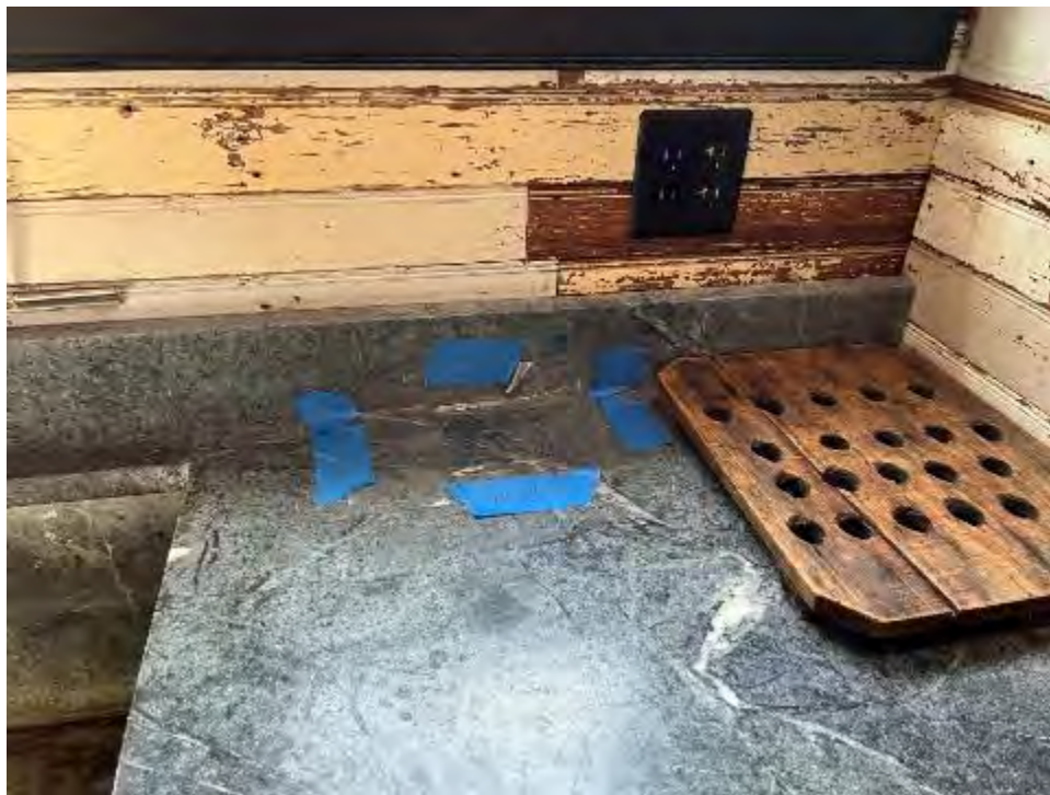
SCENE: View of wipe sample location WP-14 collected from the first floor kitchen counter.
