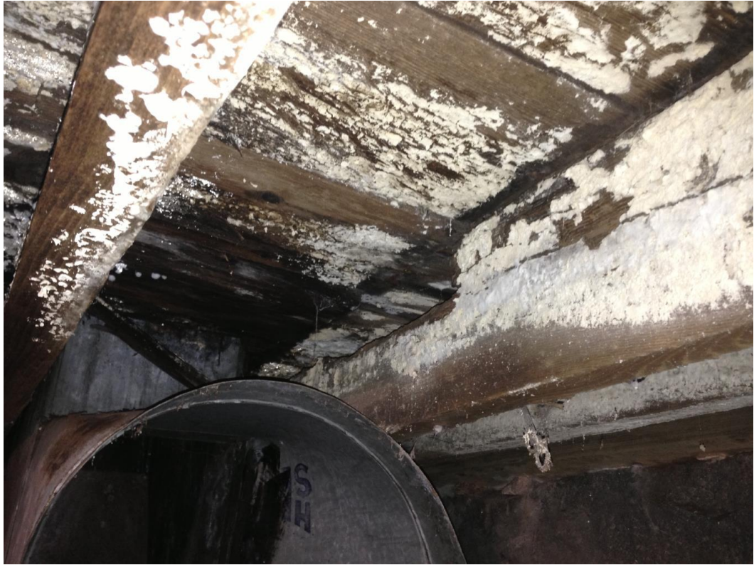
Figure 12: Wet, moldy, rotting joists and floor decking under the South Bay.
