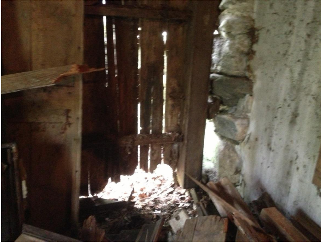
Figure 20: Hole in exterior wall as seen from the Addition Basement.
