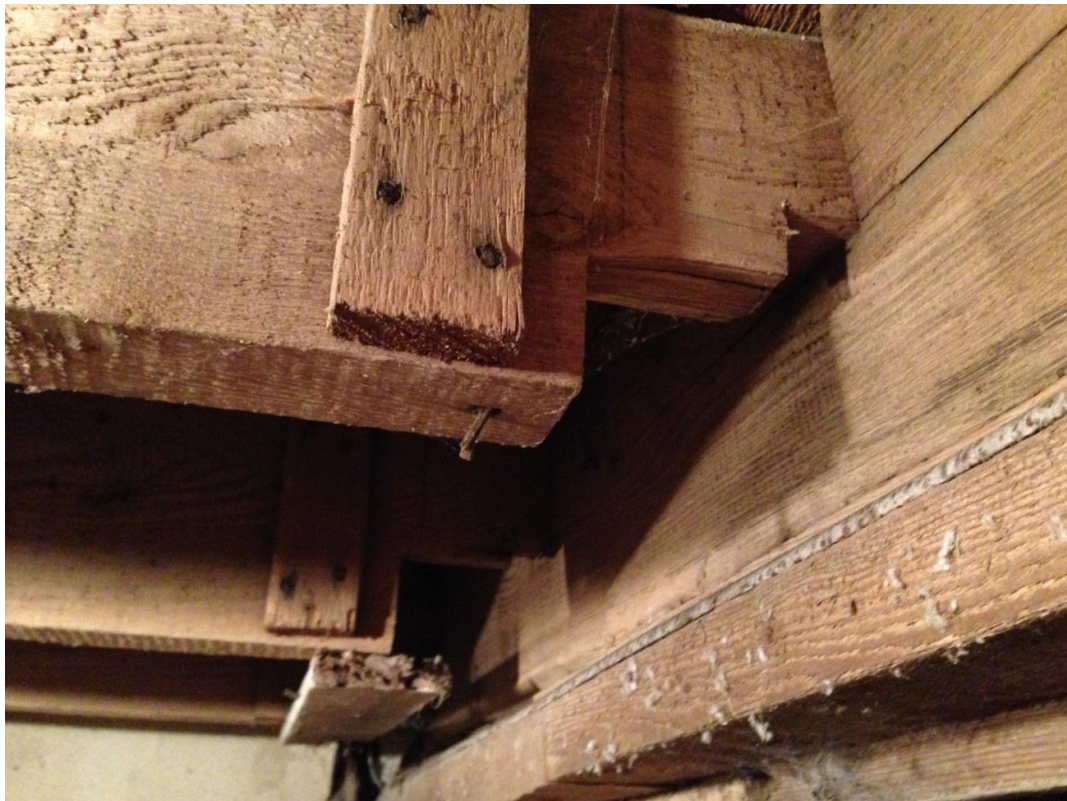
Figure 16: Crossbeams notched at the end of the spawn at the back end of the Main Building.
