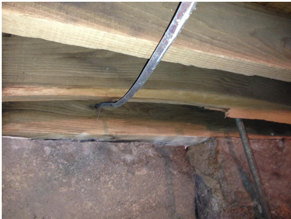
Figure 15: Warped, cut joists between Carrier Beam A and B - Front View
