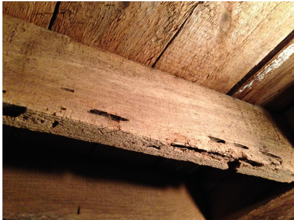
Figure 13: Decaying joist with mold on the floor decking.
