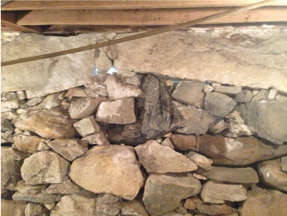
Figure 21: Hole in Western foundation wall with visible daylight.
