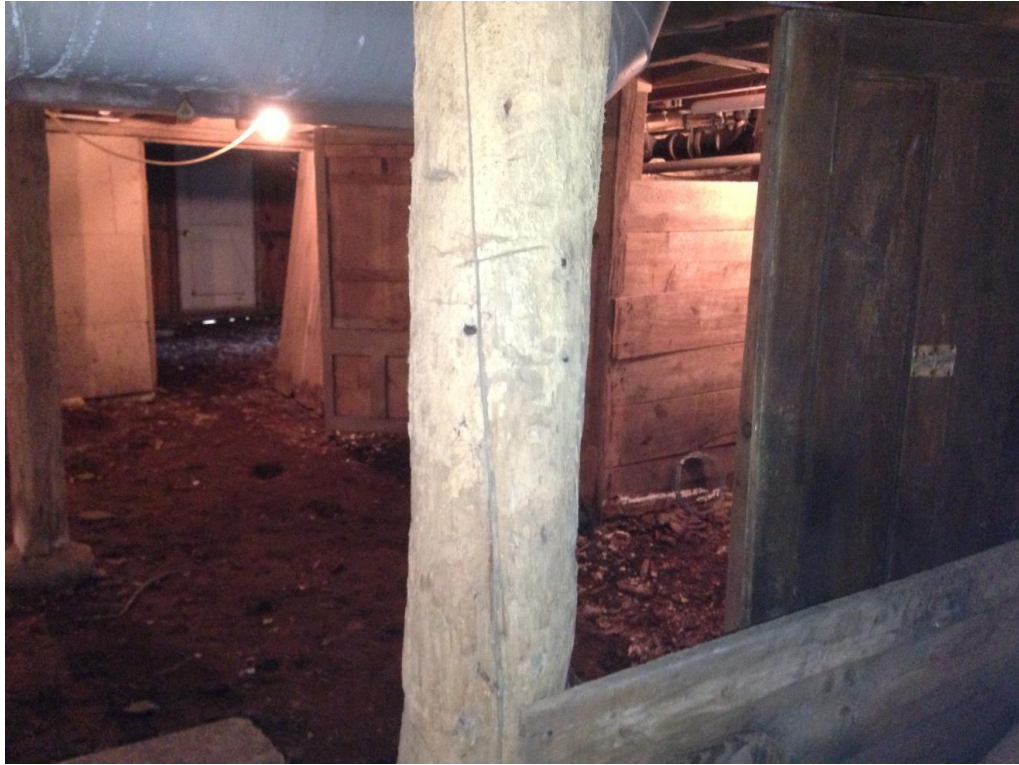
Figure 17: Basement support column splitting down the middle due to axial compression.
