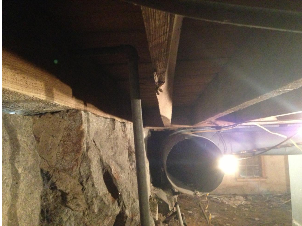
Figure 14: Warped, cut joist in between Carrier Beams A & B - Side View.
